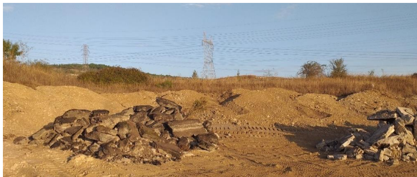
Pict. NS7.1. Site cleaning setting aside residues (asphalt) and inert material (@Vilela, CEA)
