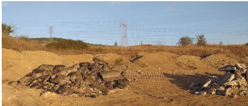
Pict. 7.1. Site cleaning setting aside residues (asphalt) and inert material (@Vilela, CEA)
